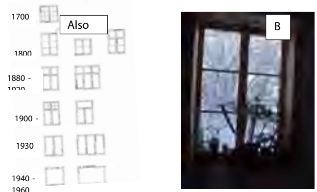
Figure 12. Window types during 1700 and 1960 [7] and B. A more modern construction from 1970, looking quite old in design and being 1.6 m high (Photo I Wästerlund).
